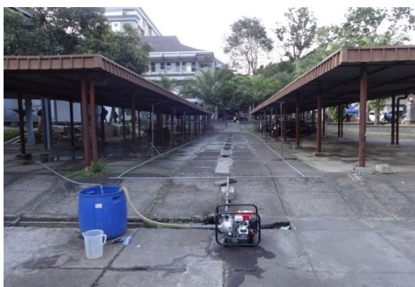
Picture 1. Sprinkler Irrigation System Installation from the Design Figure (Figure 1) in Laboratory.
